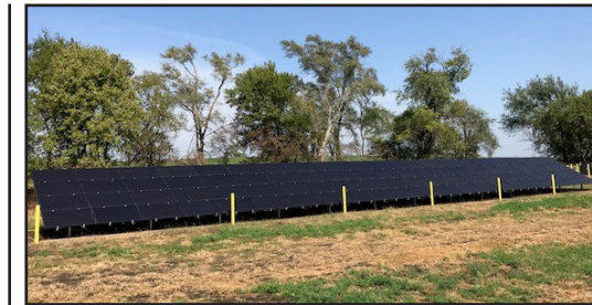
Focused Extraction Well FEW-14 Solar Array
