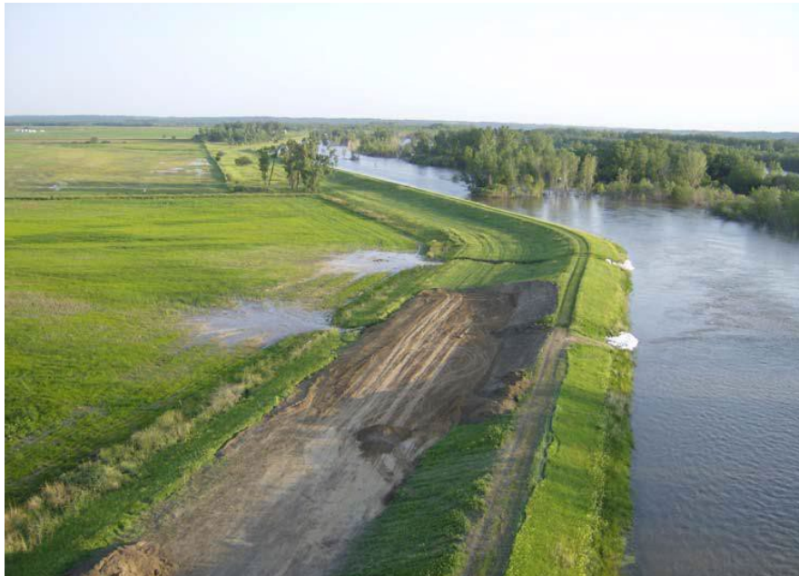
Figure 4: Damaged Levee along the Missouri River L-575 Levee System near Hamburg, IA (Photo taken June 2011, USACE Omaha District)
